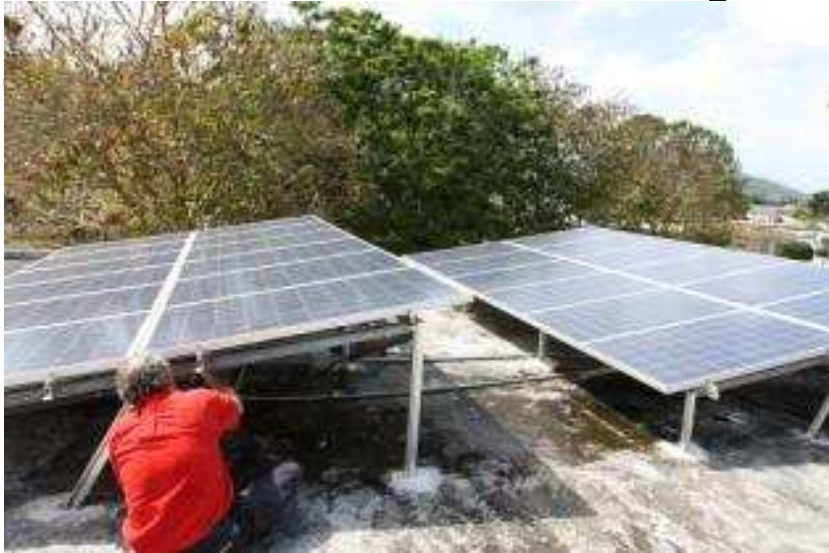
Rooftop PV Projects in the City of Caguas.
